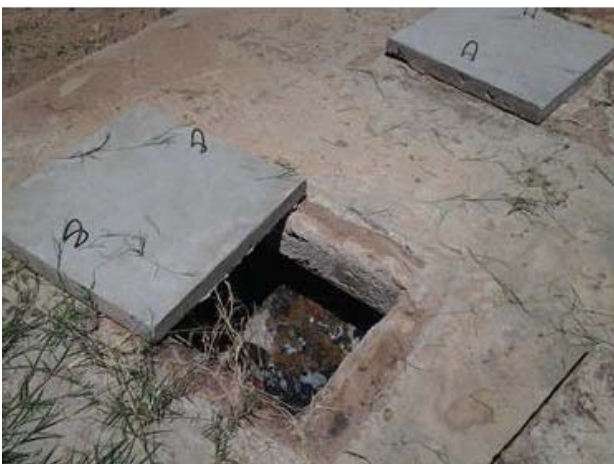
(a)Septic Tanks at A'level dormitory
