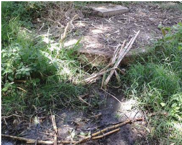
(a) Overflowing Soak away pit
