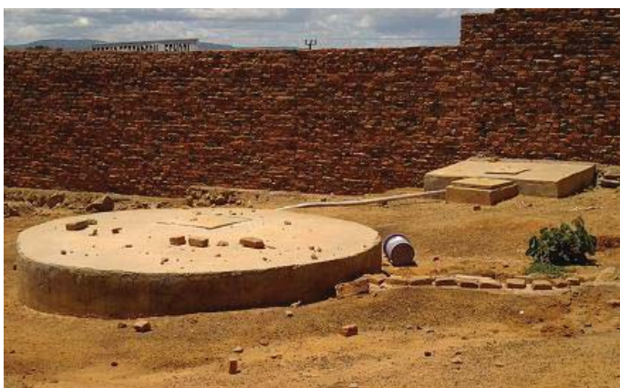
(a) Septic Tanks and Soak away Pit
