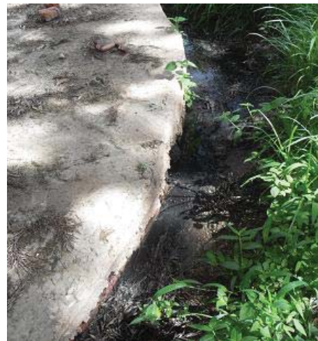
(a)Failure of a soak way pit
