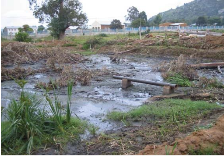
Figure 1. Conditions of failed mechanical system in Kleruu
